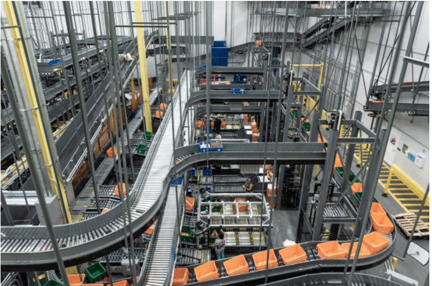
Nine miles of conveyor belts within FreshDirect's new Bronx distribution center weave through the 400,000-square-foot warehouse. PHOTO: DAVID 'DEE' DELGADO FOR THE WALL STREET JOURNAL
